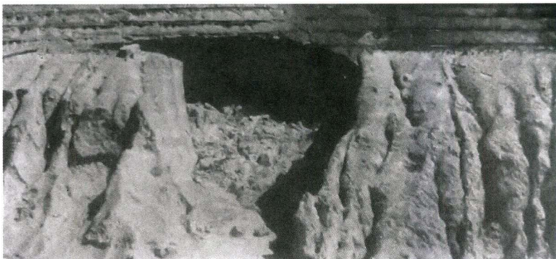
c) Landslide erosion
